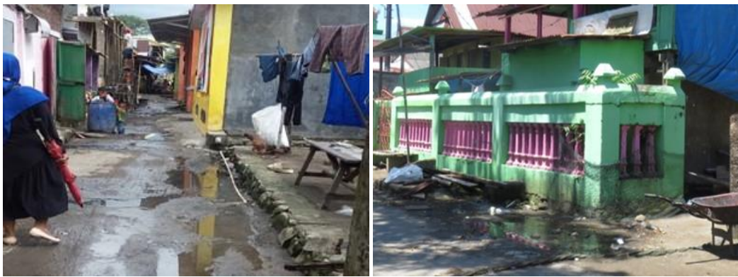
Figure 5. Street drainage condition in residential environment
