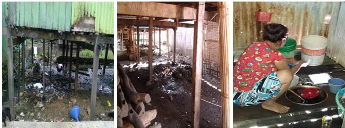
Figure 8. Drainage of the house on stilts directly throw to the kolong and the form of grey water disposal from the service area on stilt houses
